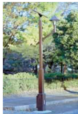
Lights powered by solar energy
